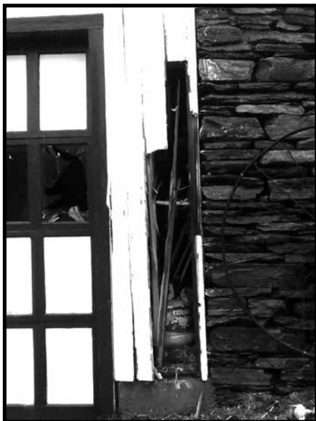
Ice House damage. Photo by Ann Letendre
