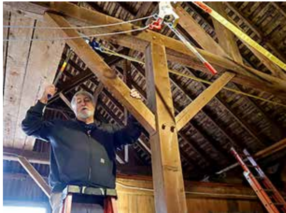
Dave Smith, also Vernon’s Town Engineer, joins other Northford Timber Framers to secure the barn roof. Dave is president of the volunteer group. To see more photos of the group working on the barn, visit the FVF Facebook page.
